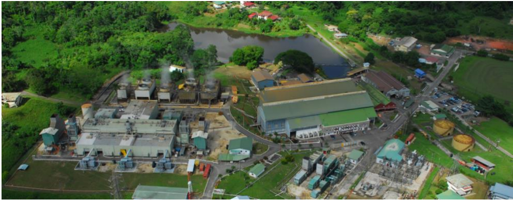
Figure 5: Powergen Penal, Trinidad & Tobago. Source Powergen
