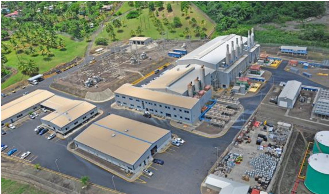
Figure 4: Cul De Sac Power Station, Saint Lucia. Source: LUCELEC
